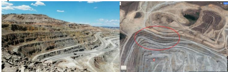
Figure 9. 2017.6 months - lateral slope, partial collapse / also soil 5 stack / and probable partial mine pressure
